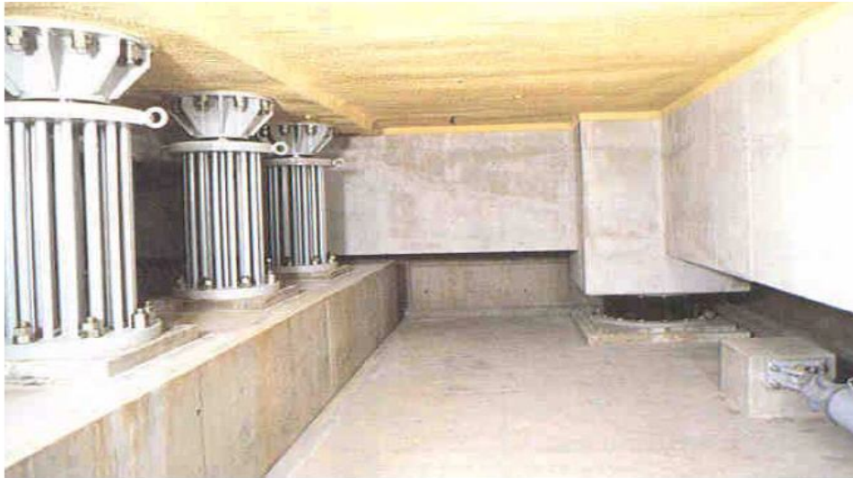
Isolation devices of Bridgestone Toranomon Building
