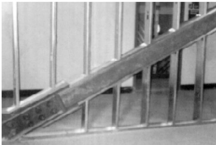
Pall friction-damper at bottom of single diagonal brace
