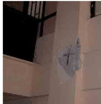
Mortar is fallen down. There was no cover concrete initially, so the reinforcing bars are exposed easily, but there is almost no cracks in concrete.
