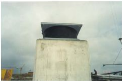
High damping rubber bearing just installed in the apartment houses of IERP at Città di Castello (Perugia), as filmed in May 2001.
