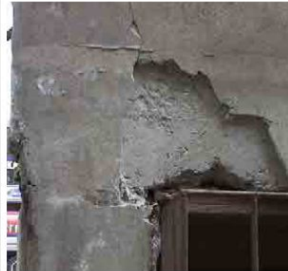
Only flexural cracks occur in beam
