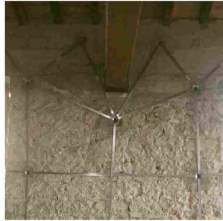
Detail of the link to the R/C kerb around a wooden truss.
