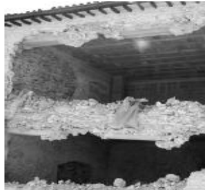
Out of plane collapse of a bearing wall roof and bad connection tie beam-wall
