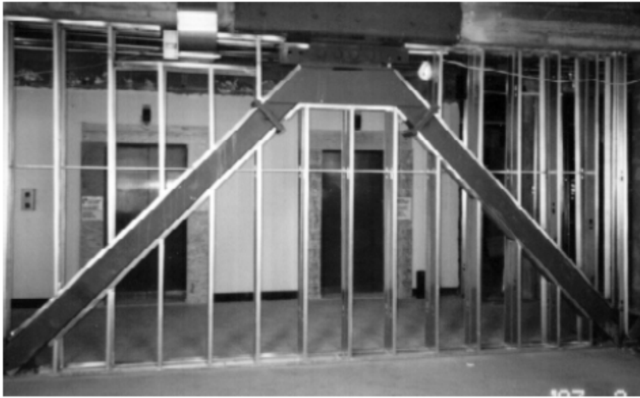
Pall friction-damper at top of chevron brace
