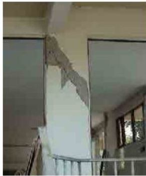
Big shear crack at the top of column
