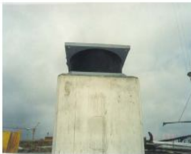
High damping rubber bearing just installed in the apartment houses of IERP at Città di Castello (Perugia), as filmed in May 2001.
