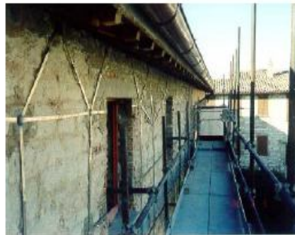
Application of the CAM method to the seismic improvement of a masonry apartment building at Sigillo (Perugia) (filmed during works in December 2000).
