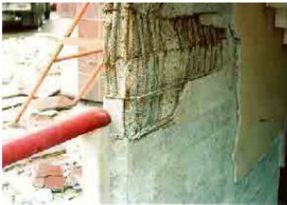
Tensile crack at the middle height of column
