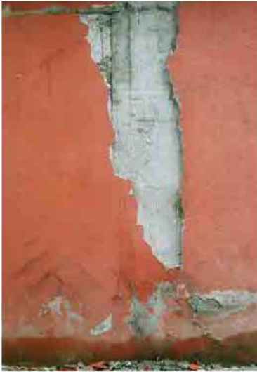
Mortar is separated and fallen down, and No shear cracks are observed
