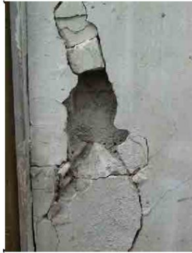
Big crack is observed on mortar. But take the mortar away, no crack is observed on the face of concrete.
