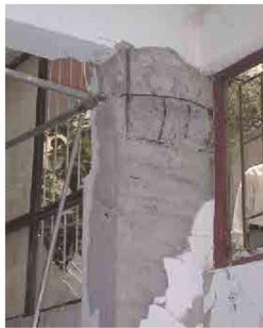
Buckling of reinforcing bars Crush of core concrete
