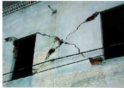
Diagonal cracks observed
