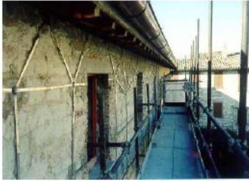
Application of the CAM method to the seismic improvement of a masonry apartment building at Sigillo (Perugia) (filmed during works in December 2000).
