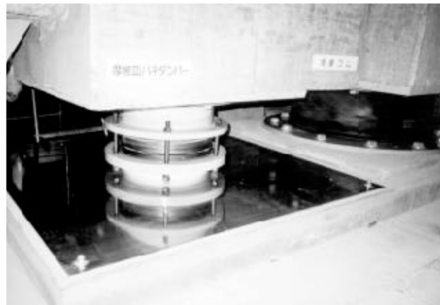
Photo of the friction damper with the coned disc springs in the actual base-isolation building
