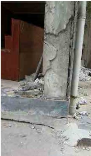
Corner cover concrete is spalled off. But shear cracks are not observed.
