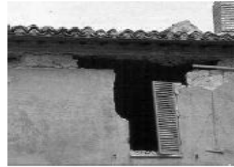
Partial collapse due to the thrust of the
