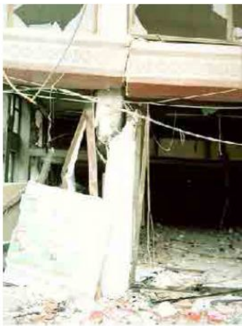
Buckling of reinforcing bars Visible settlement and/or inclination of floor
