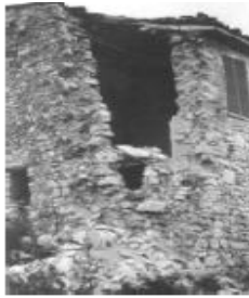
Failure of a building corner
