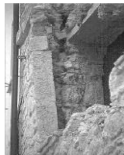
Eccentric loading to concrete tie positioning
