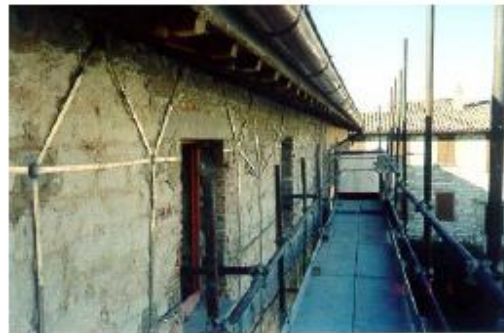
Application of the CAM method to the seismic improvement of a masonry apartment building at Sigillo (Perugia) (filmed during works in December 2000).
