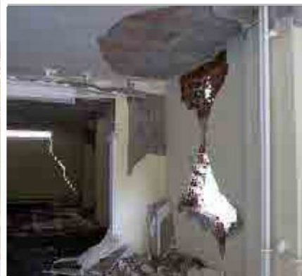
Extensive diagonal cracks penetrated and Offset from RC frame
