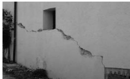
Shear failure of a wall
