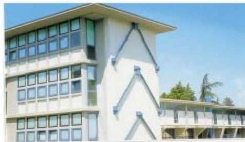
Visco-elastic dampers installed in the Gentile Fermi school at Fabriano (a rare example of rationalist architecture), during seismic improvement works (filmed in 2001).
