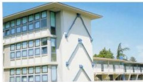
Visco-elastic dampers installed in the Gentile Fermi school at Fabriano (a rare example of rationalist architecture), during seismic improvement works (filmed in 2001).
